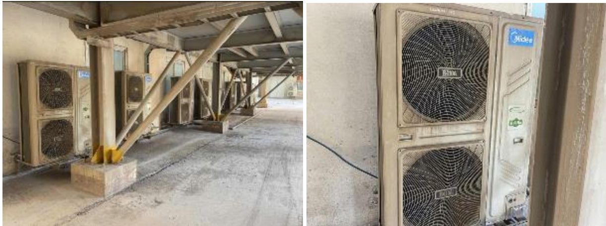
Figure 4.20. Local air conditioning systems are installed in areas around the factory.
