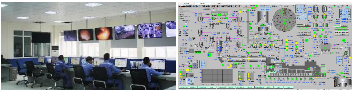
Figure 4.27. Monitoring and control operations at the Cement Plant Control Room & LINES system interface with high operational data density.
