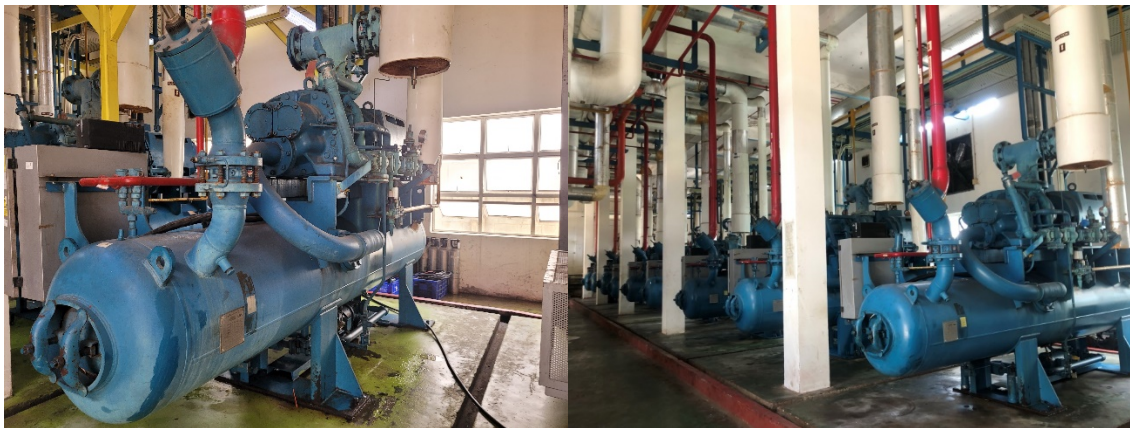
Figure 4.6 Screw refrigeration compressors at the facility
