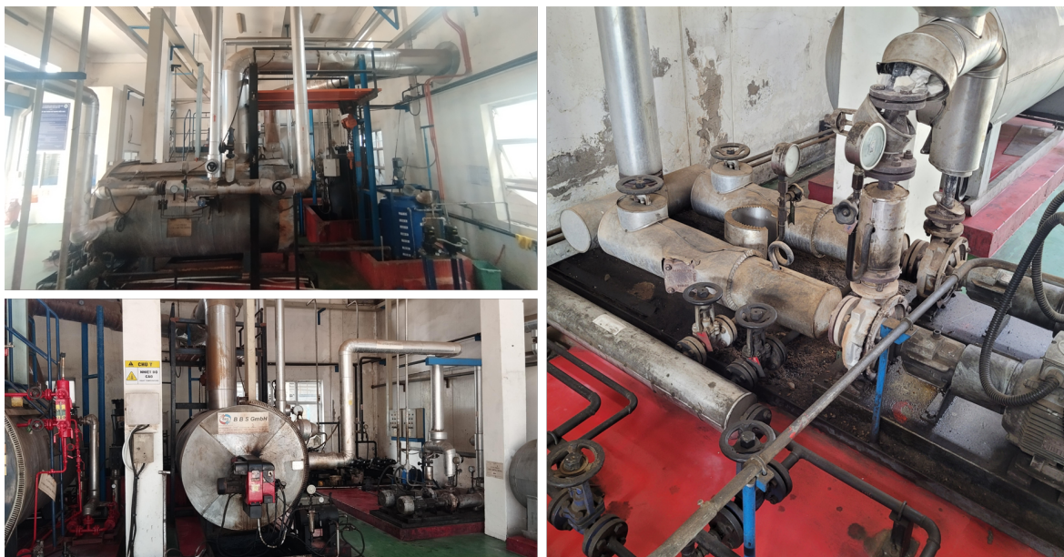
Figure 1.12. Thermal oil heater and oil pumping system
