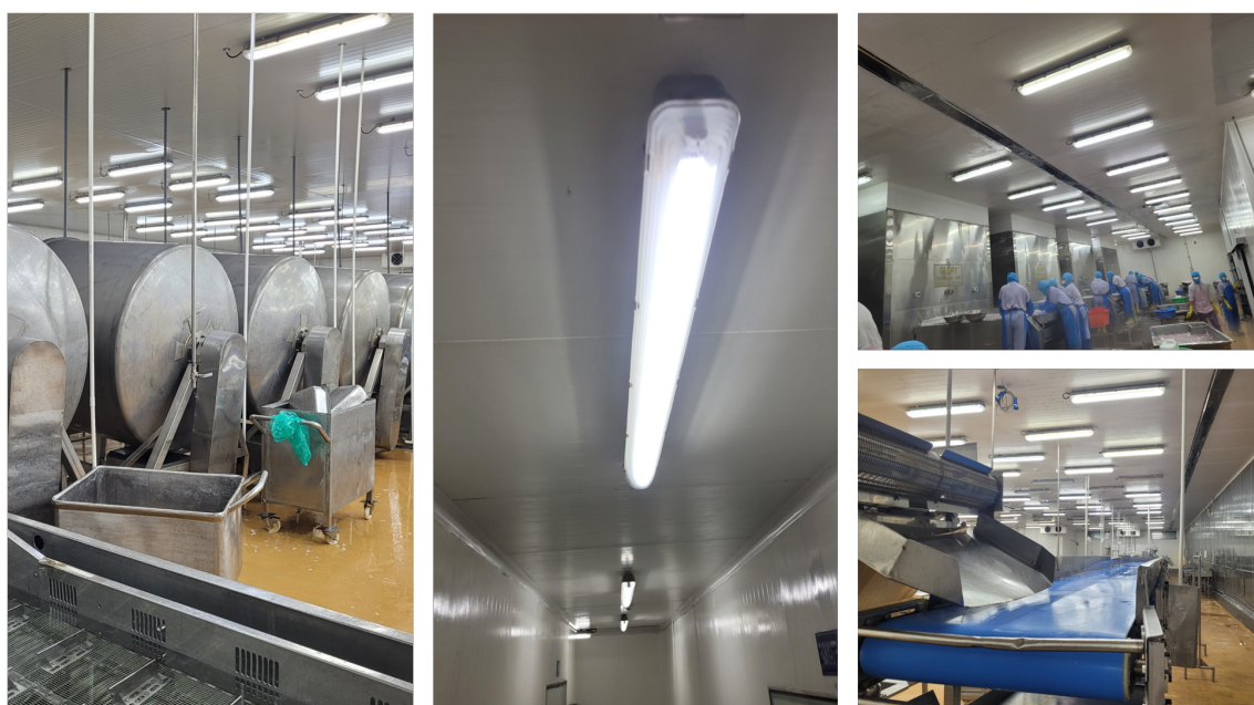
Figure 1.7. Lighting system at the factory
