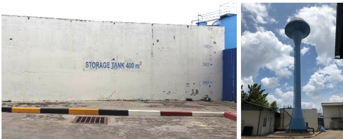
Figure 1.15. Factory's water storage tank and water tower system
