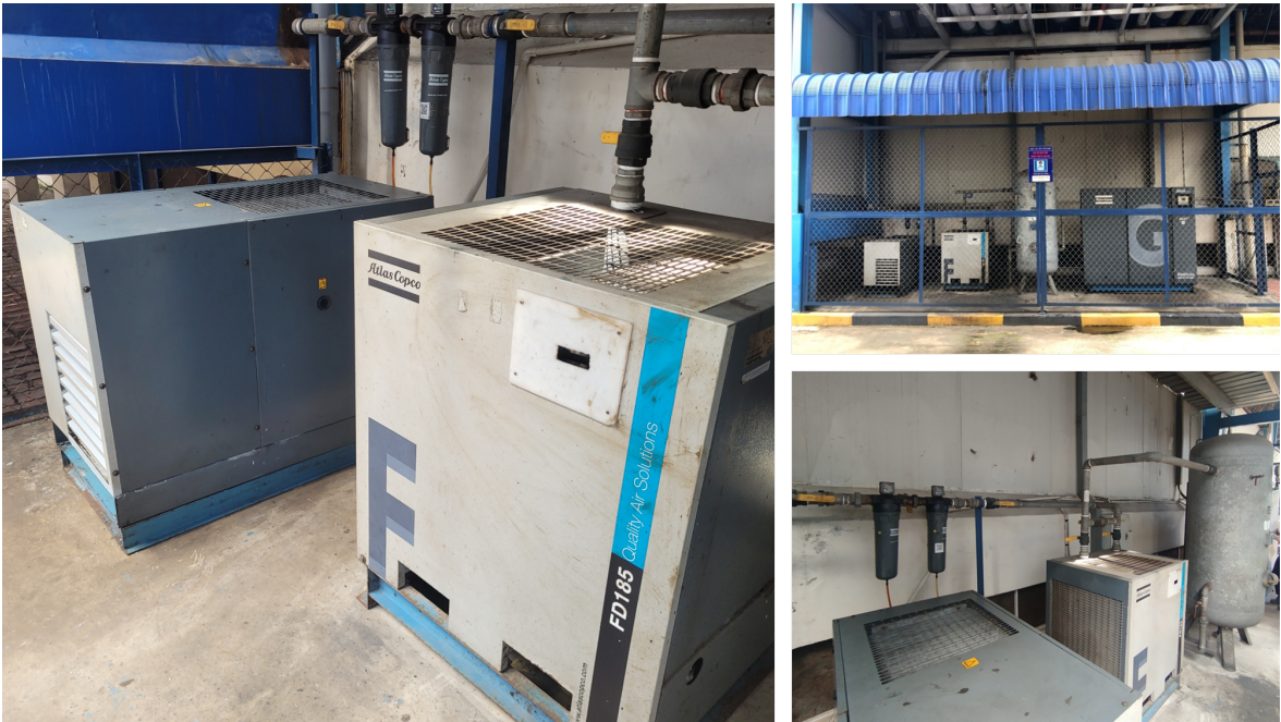
Figure 1.8. Compressed air system
