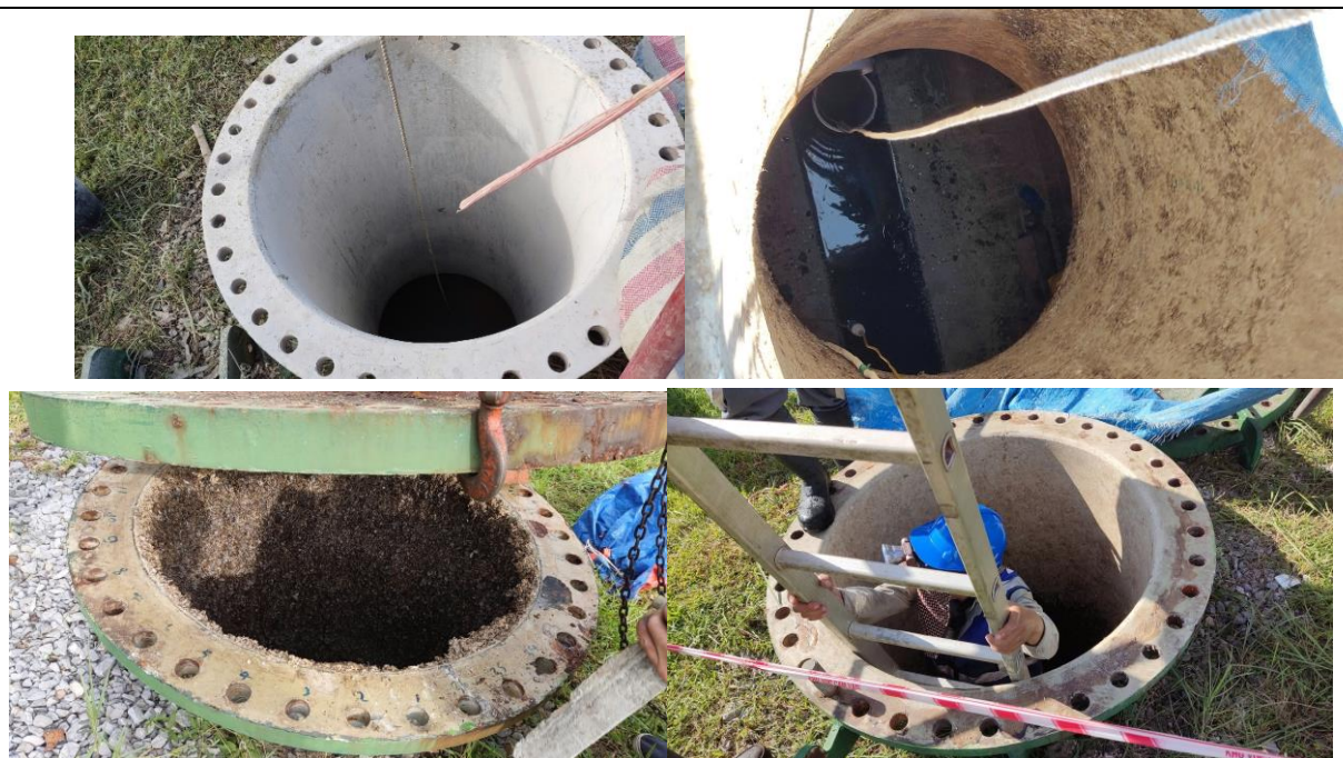
Figure 4.8. Actual Images of the Manholes
