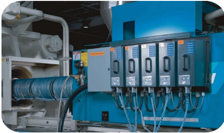
Figure 8: Replace the cylinder barrel heating system for the plastic injection molding machine
