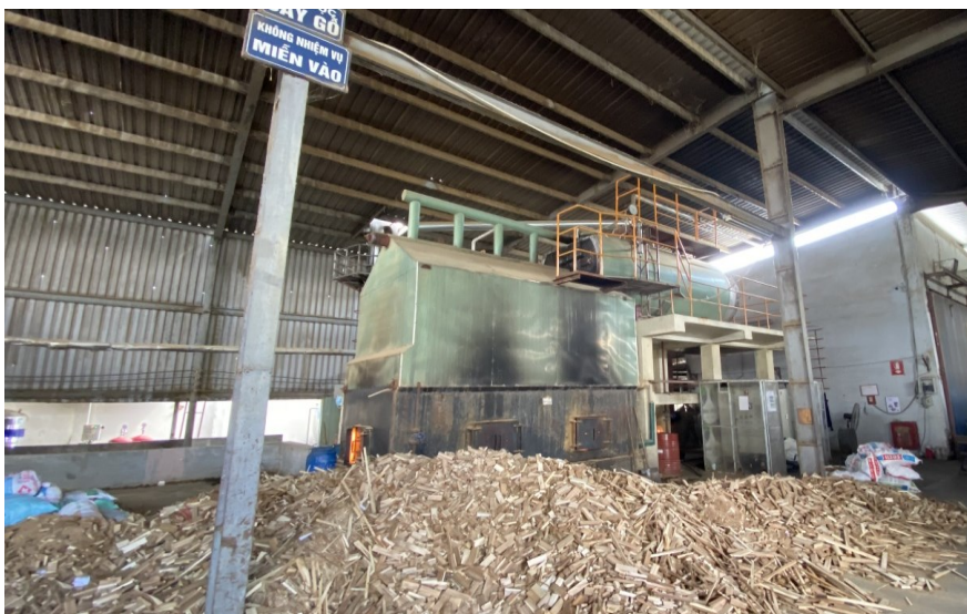
Figure 4. Example of boiler installation in Vietnamese wood processing industry
